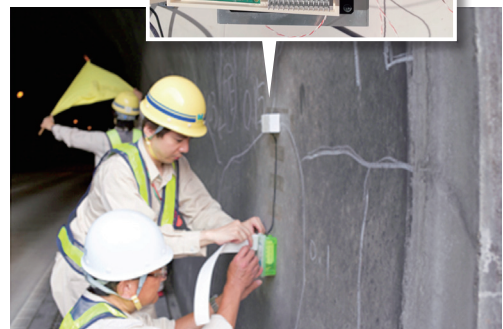
Demonstration of monitoring devices in a tunnel
