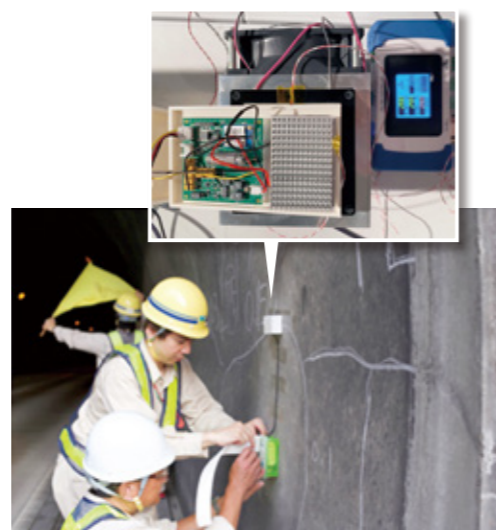
Demonstration of monitoring devices in a tunnel
