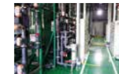
Initiative by Dalian Seiko Instruments Inc.: Investment in state-of-the-art factory wastewater treatment facility
